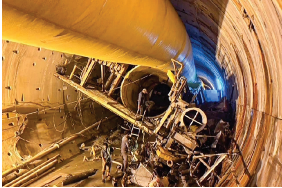
Rescue operation underway to trace workers trapped inside the partially collapsed Telangana's Srisailem Left Bank Canal tunnel, in Nagarkurnool on Saturday
