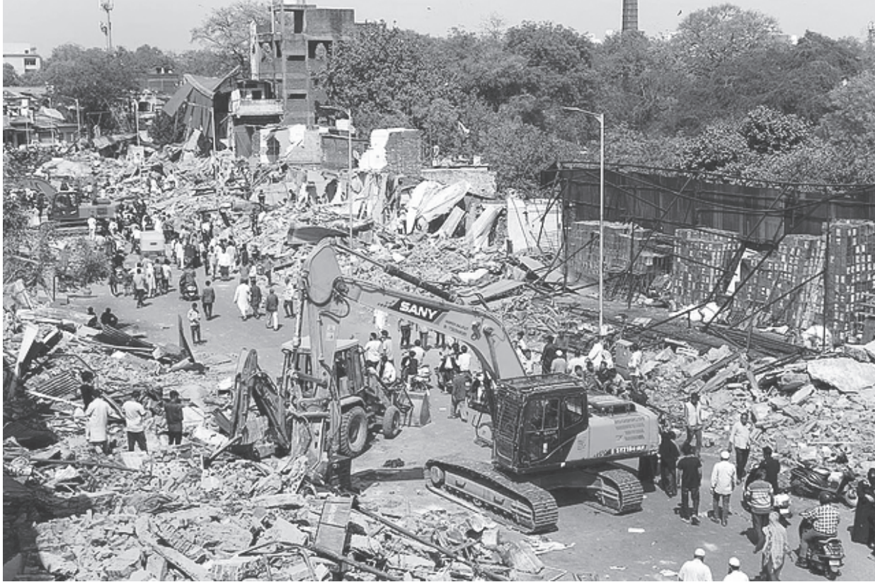
Earthmovers demolish illegal encroachments along a road during an anti-encroachment drive by Ahmedabad Municipal Corporation (AMC), in Ahmedabad, Gujarat on Saturday.
